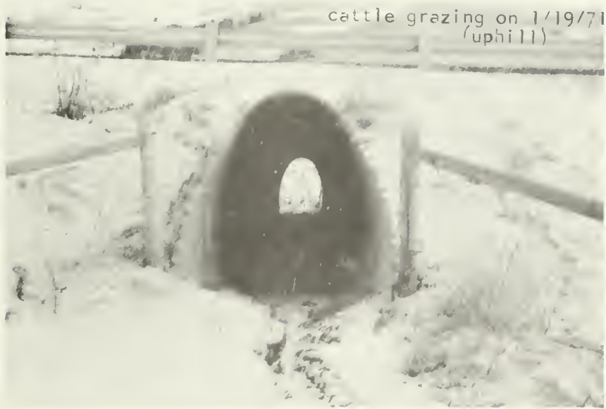
EAST ENTRANCE Notice drainage from upper draw
